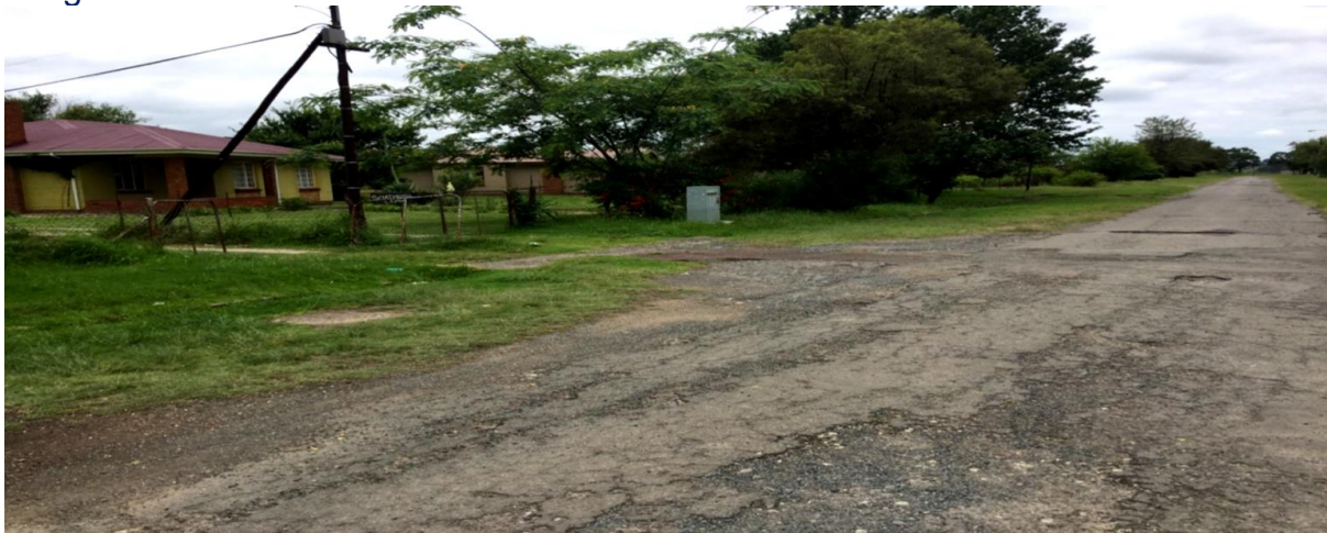
Image 2: Unrehabilitated Urban Tarred Road.2
