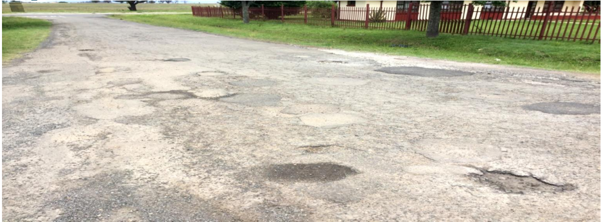
Image 1: Unrehabilitated Urban Tarred Road.1
